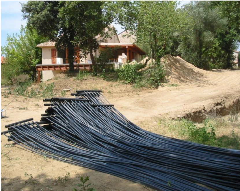
Colector horizontal, geopanel
