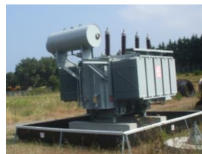
BSTP 30000 litros (EDF France)
